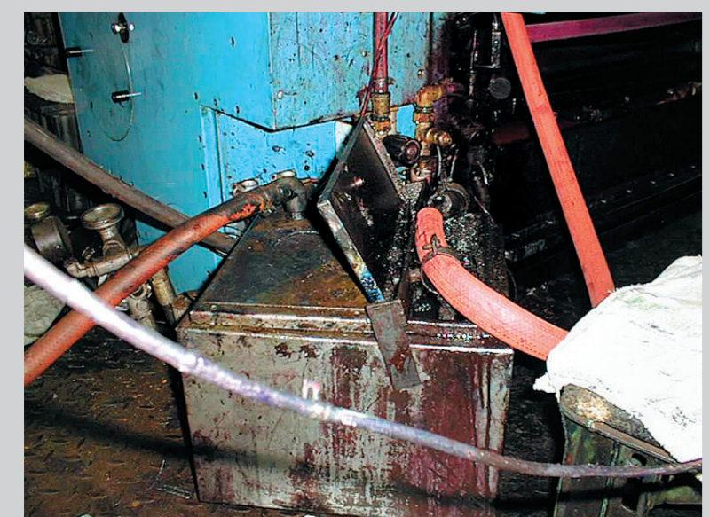
Overload of a poorly maintained intermediate tank. Photo Technotrans.
